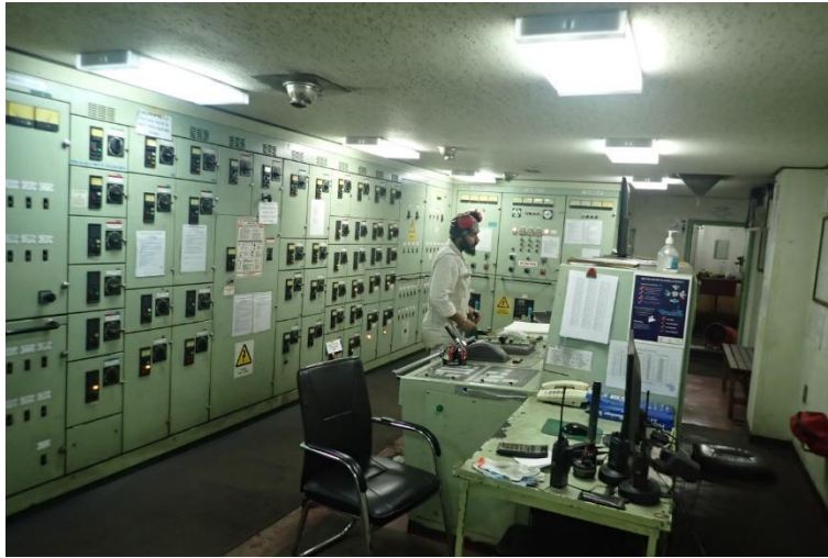
Engine control room
